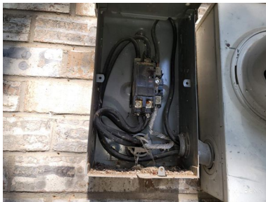
Condenser disconnect panel
