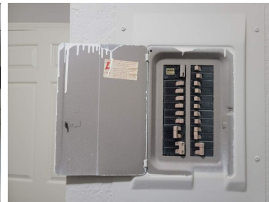
Main breaker panel
