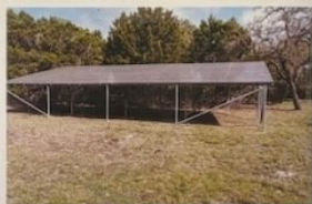
30545 Bridlegate CPS Electricity Cost (including solar connection fee)
